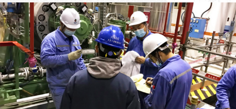
→ HYHNPC has developed and implemented a plan and put Unit 5 into operation accordingly on schedule. Its annual power generation was 8.2% higher than the annual target in 2021, effectively alleviating power shortage in Northeast China.
