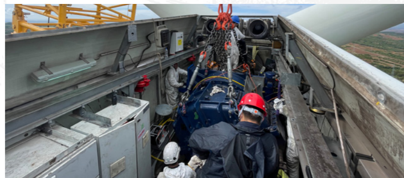
→ In Changgao Wind Farm, Liaoning Province, the GE2MW gearbox is utilized for the first time in China, solving the problem of long shutdowns of the unit and generating 1 GWh of electricity.
