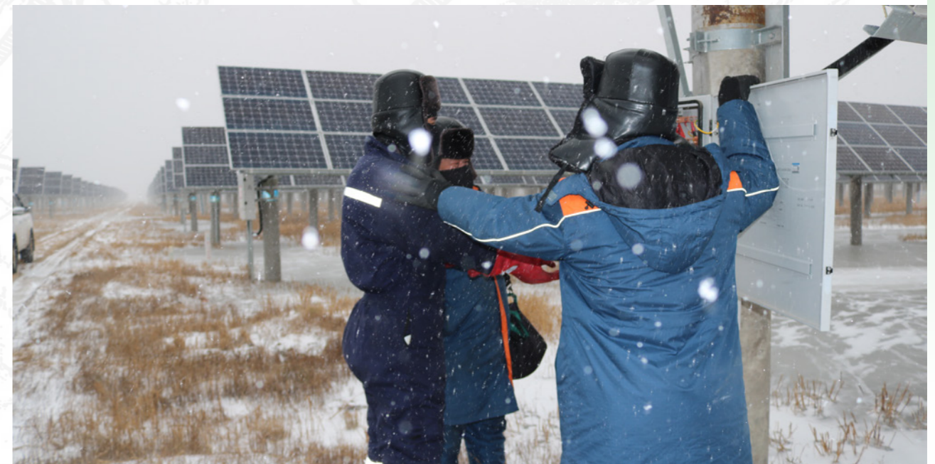
→ In Zixing Solar Farm, Jilin Province, employees conduct special inspections on the PV panels to check the tightness of the component brackets to ensure their normal operation.
